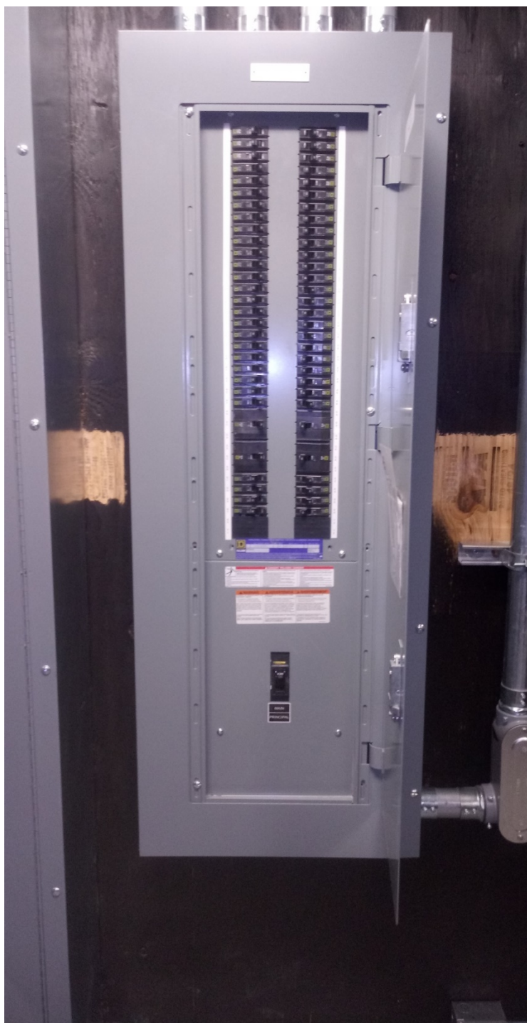
Server Room 122 – Panel UPS labeling.
