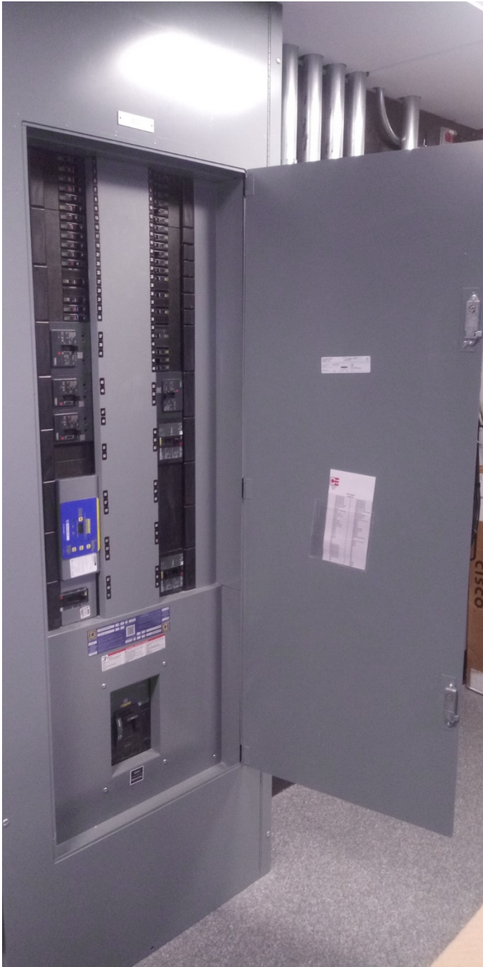
Server Room 122 – Panel ECC labeling.
